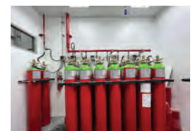
Automatic fire suppression system NOVEC 1230
