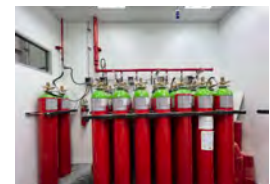
Automatic fire suppression system NOVEC 1230
